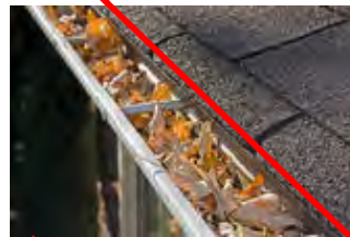
gutter not clean
